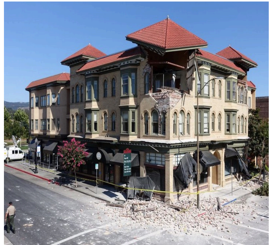
A building downtown at 2nd and Brown sustained damage from the 6.0 earthquake in Napa. (Steve Rhodes/Demotix/Corbis)
