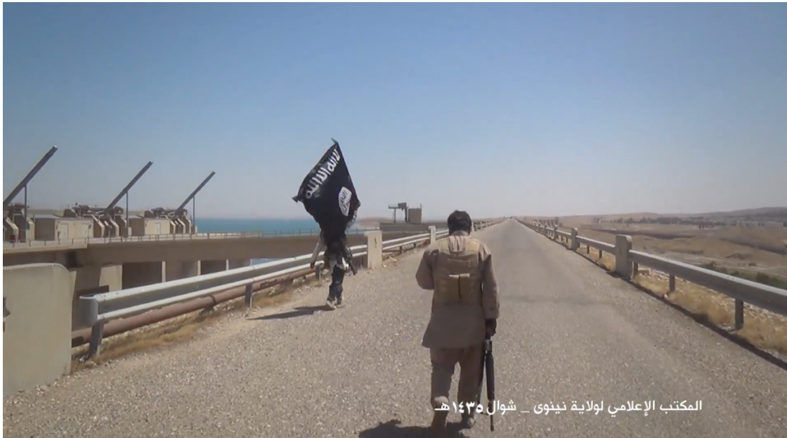
Figure 6.6: Screenshot from video entitled "Tour Of Liberated Territories - Mosul Dam And Shingal" (Wilayat Ninawa, 2014) where IS fighters are walking over one of the headworks of Mosul Dam.
