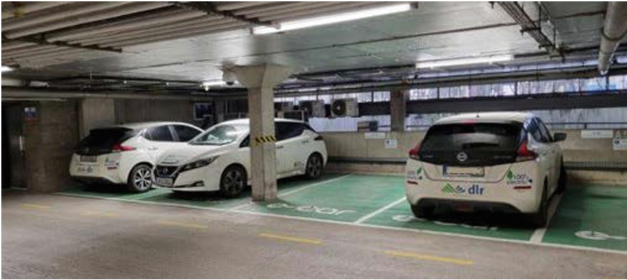
Fig. 4. Current EV charging facilities located in the County Hall basement. Image courtesy of UCD and DLR,
